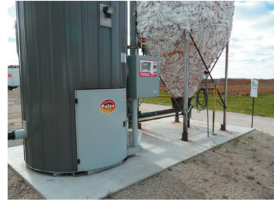
Pelco boiler and fuel hopper
