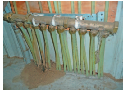
Radiant floor heat system
